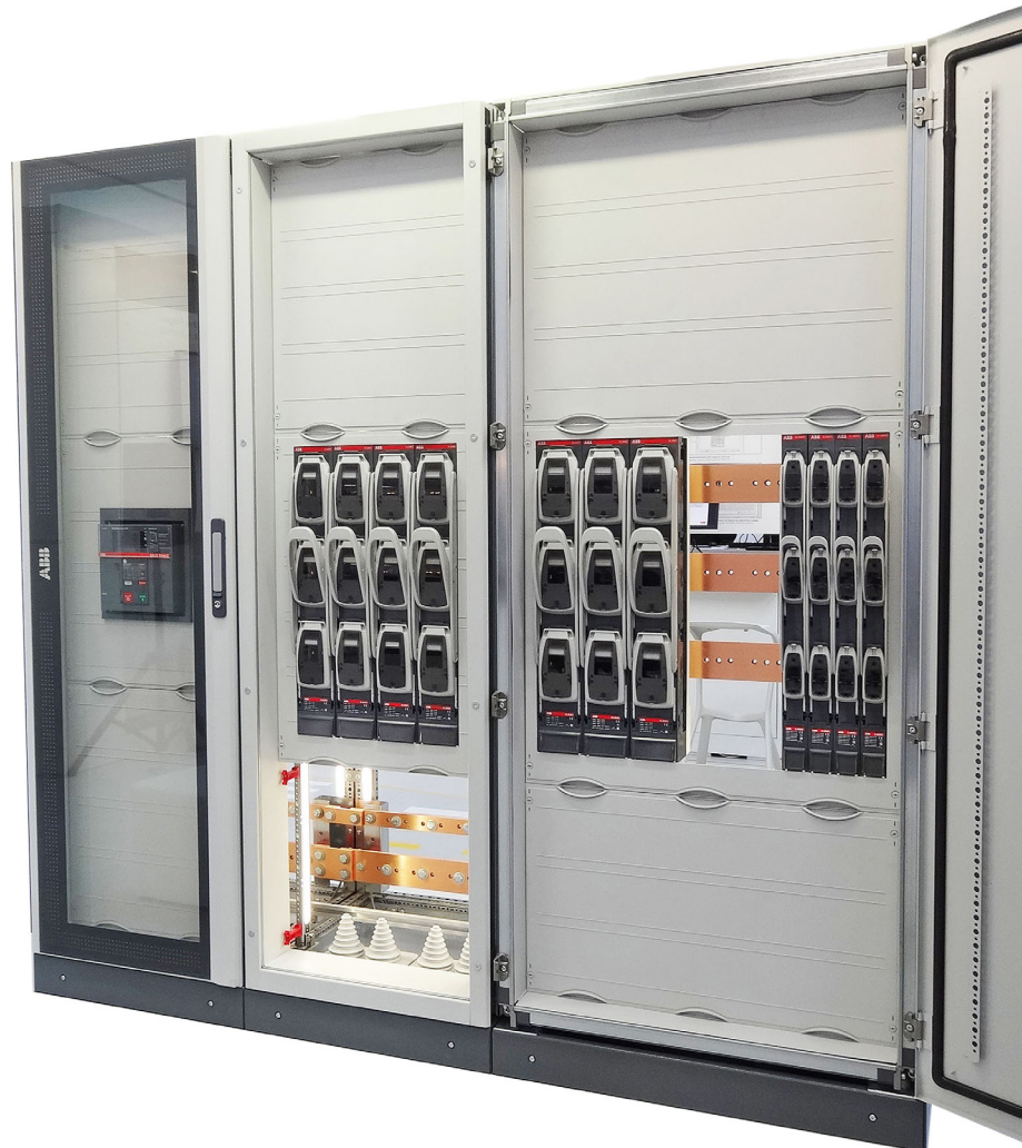
InLine II in proE power switchboard
